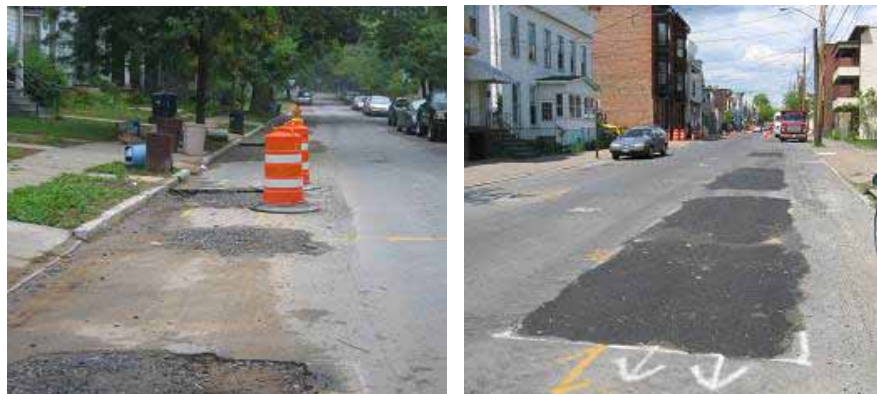
Examples of traditional service excavations/ reinstatement referred to as a "checkerboard pattern" by the LA.
